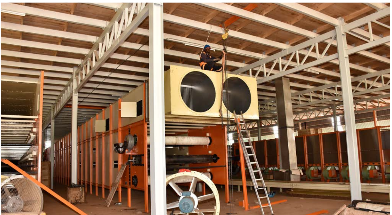
A continuous withering unit being installed at Motigo Tea Factory. Factories are adopting new technologies to improve quality and efficiency
